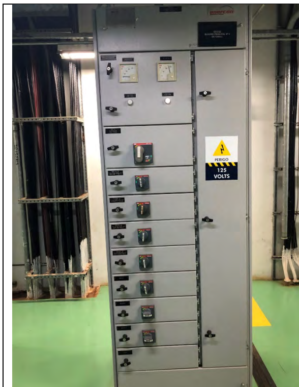
QCCG2 – Quadro principal 2 de corrente contínua
