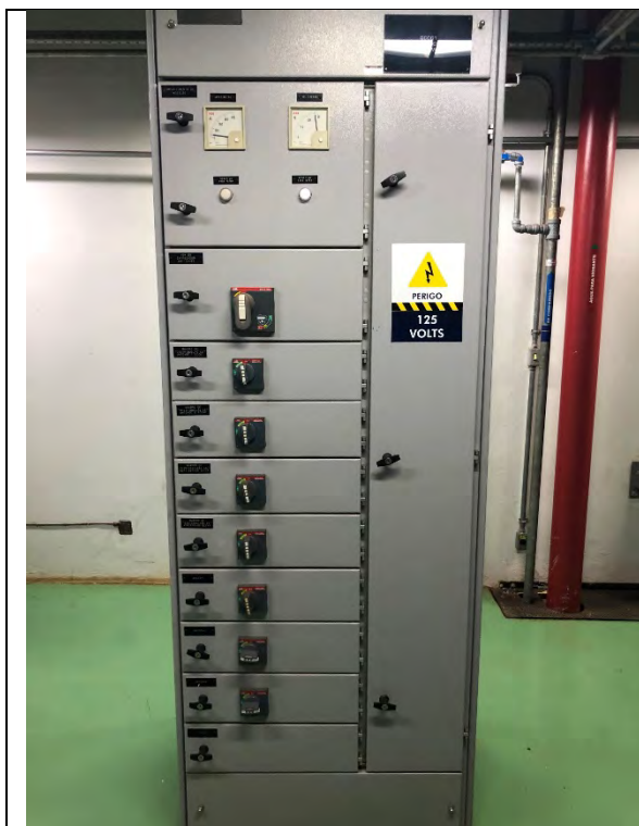
QCCG1 – Quadro principal 1 de corrente contínua
